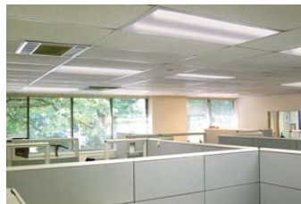
Legacy Fluorescent Lighting
