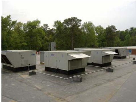
Typical Air Handler Units
