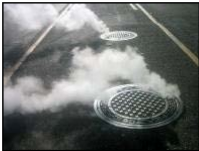
Leaking Traps Waste Energy
