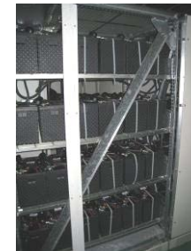
Uninterruptible Power Supplies
